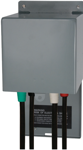
Front View with Cable Attached and Door Open
