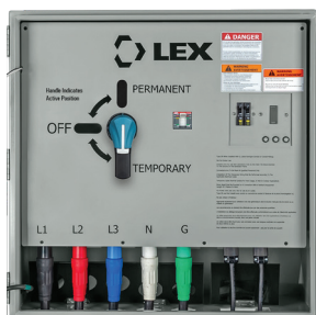
Service Entrance Rated
