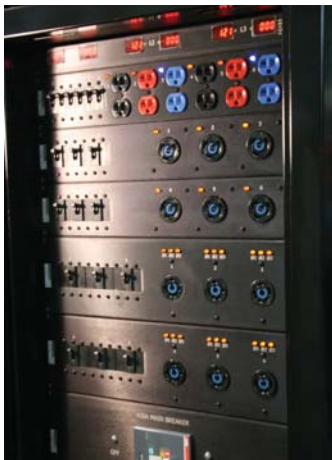
Custom 20 RU rack with locking receptacles.
